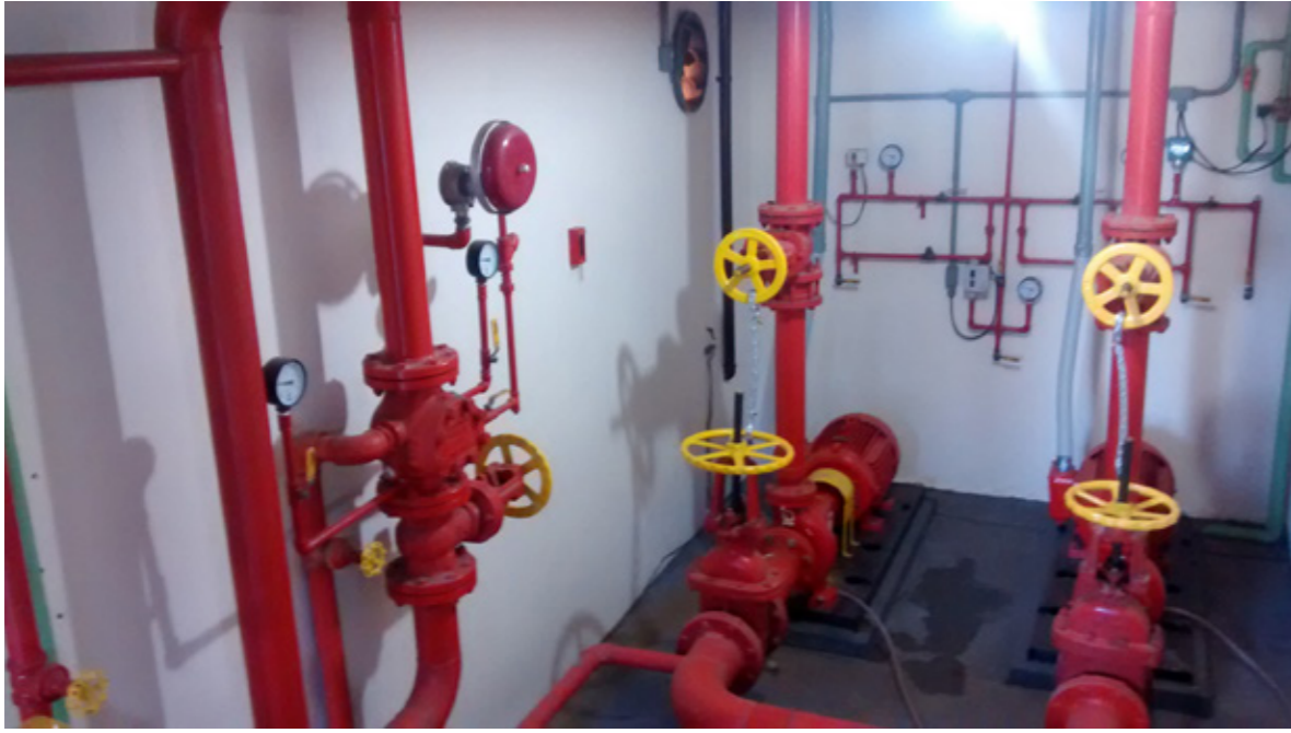
Pumps for the Fire fight system - under the TTC building
