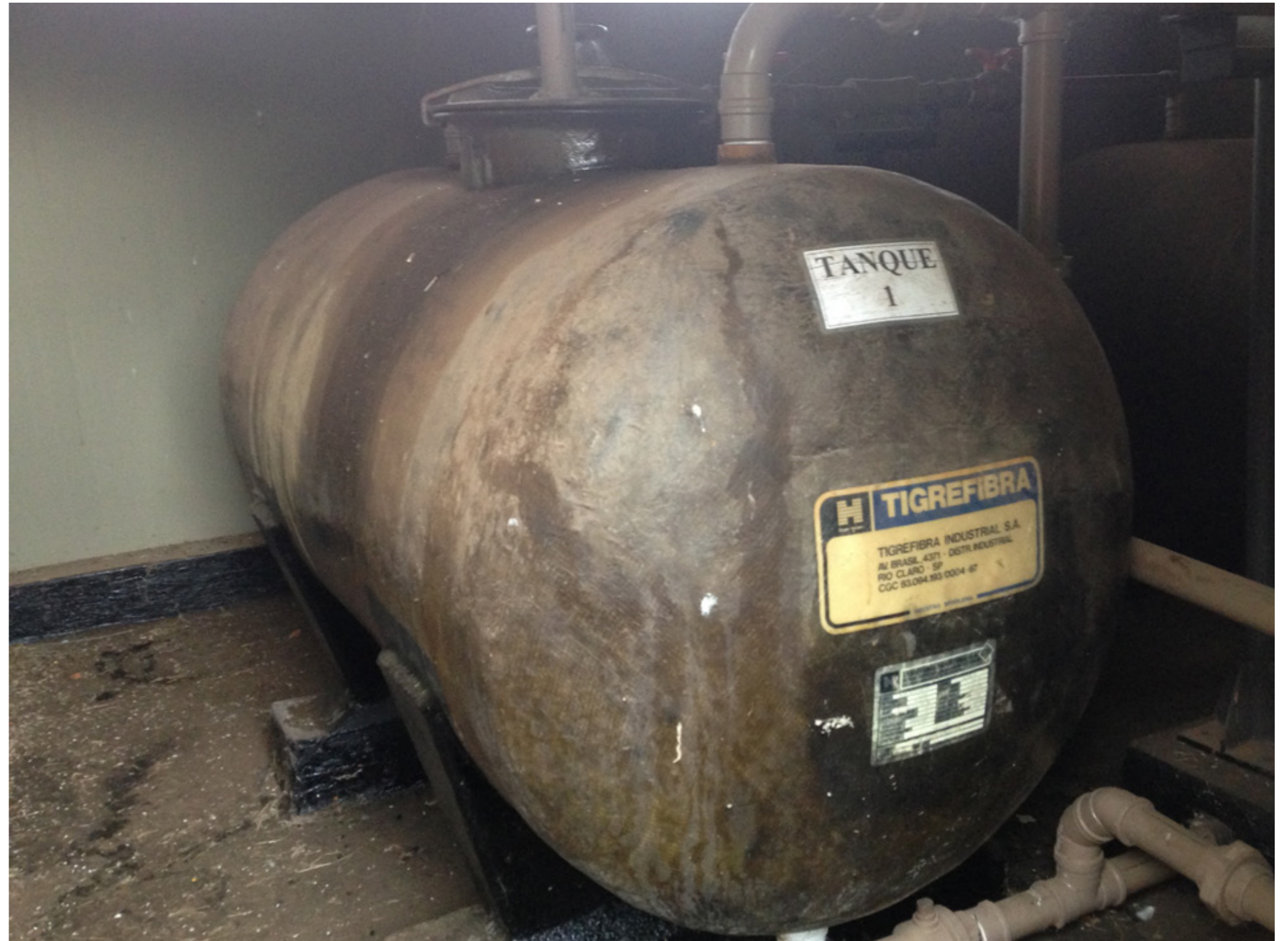
Waste Water System
